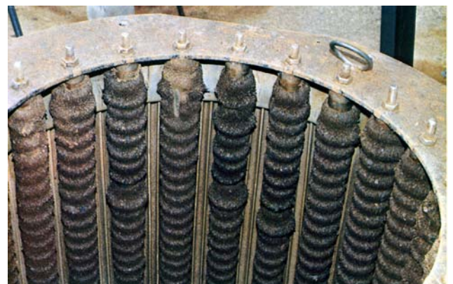
Inside view of the filter
